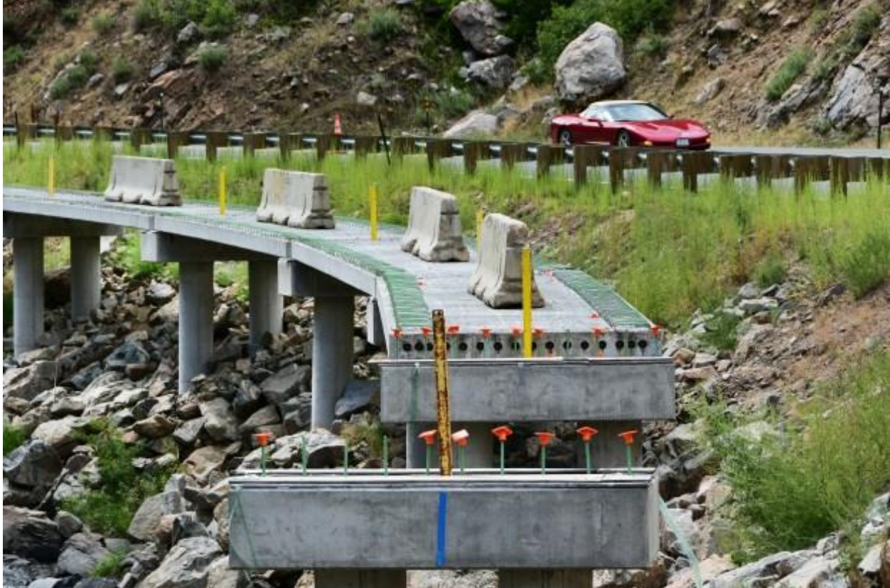
Casted concrete beams are installed for the under-construction Clear Creek Canyon trail in Jefferson County on Wednesday, Aug. 14, 2024. (Photo by Hyoung Chang/The Denver Post)
