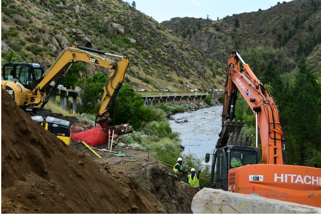
Construction continues on the Clear Creek Canyon trail in Jefferson County on Wednesday, Aug. 14, 2024. (Photo by Hyoung Chang/The Denver Post)
