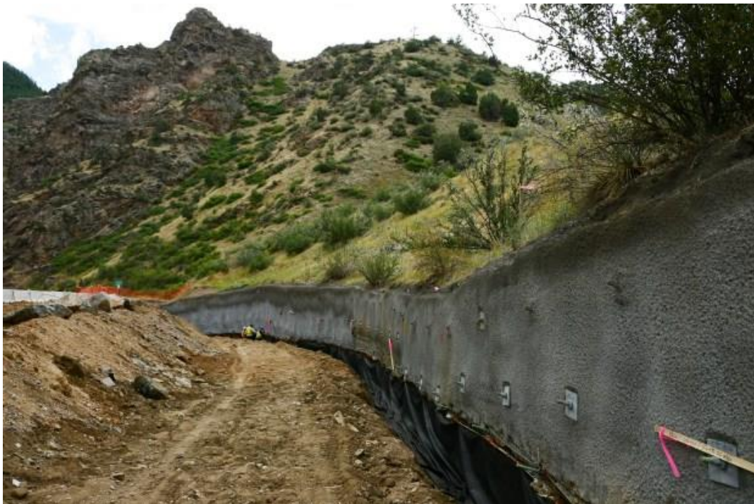
Shotcrete covers walls of the Huntsman Gulch area in Clear Creek Canyon amid trail construction in Jefferson County on Wednesday, Aug. 14, 2024. (Photo by Hyoung Chang/The Denver Post)
