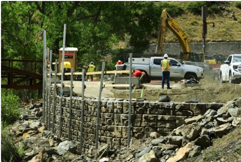
Construction is underway on one of the nine bridges for the Clear Creek Canyon trail between tunnels 5 and 6 in Jefferson County on Wednesday, Aug. 14, 2024. (Photo by Hyoung Chang/The Denver Post)
